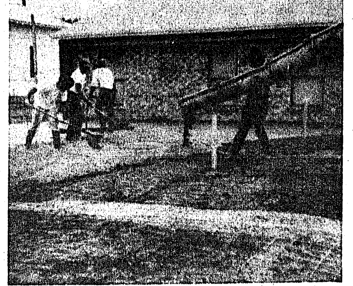
The cement slab foundation was poured Tuesday for the beginning of construction of a new addition to Cordero Baptist Church.
