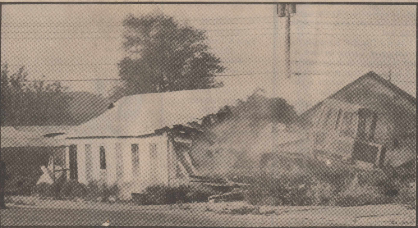
A CLOUD OF DUST: The old Rotan Tourist Courts, directly East of the Tom Collins building in Rotan, were demolished last Monday morning. The property was acquired by the Rotan School District through a tax sale and in all probability will be turned into a parking lot. The destruction of the building took approximately 20 minutes. It was a combined effort of Rotan City personnel, and workers from Fisher County Precinct 2 & 3. It certainly improved the appearance of the downtown area as will the recently completed construction of the Veteran's Park just West of Casa Morales Restaurant.
