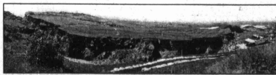
A shot of the collapsed 18th hole at Ocean Trails Golf Club.
