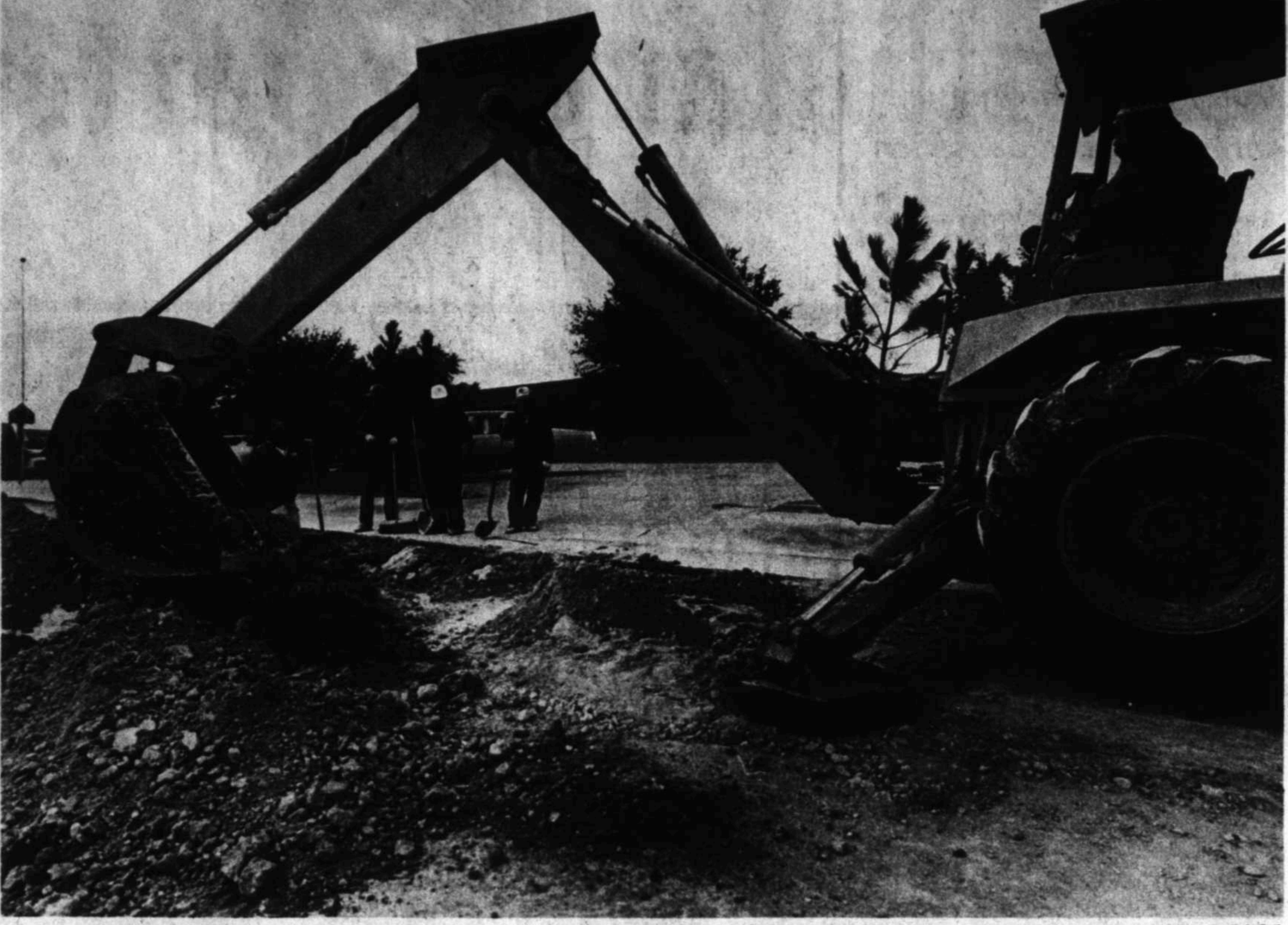
Workers stand in the background, waiting for the machine to finish installing a new water line. This is one part of a $6 million package of water and sewer improvements being implemented by the city.
