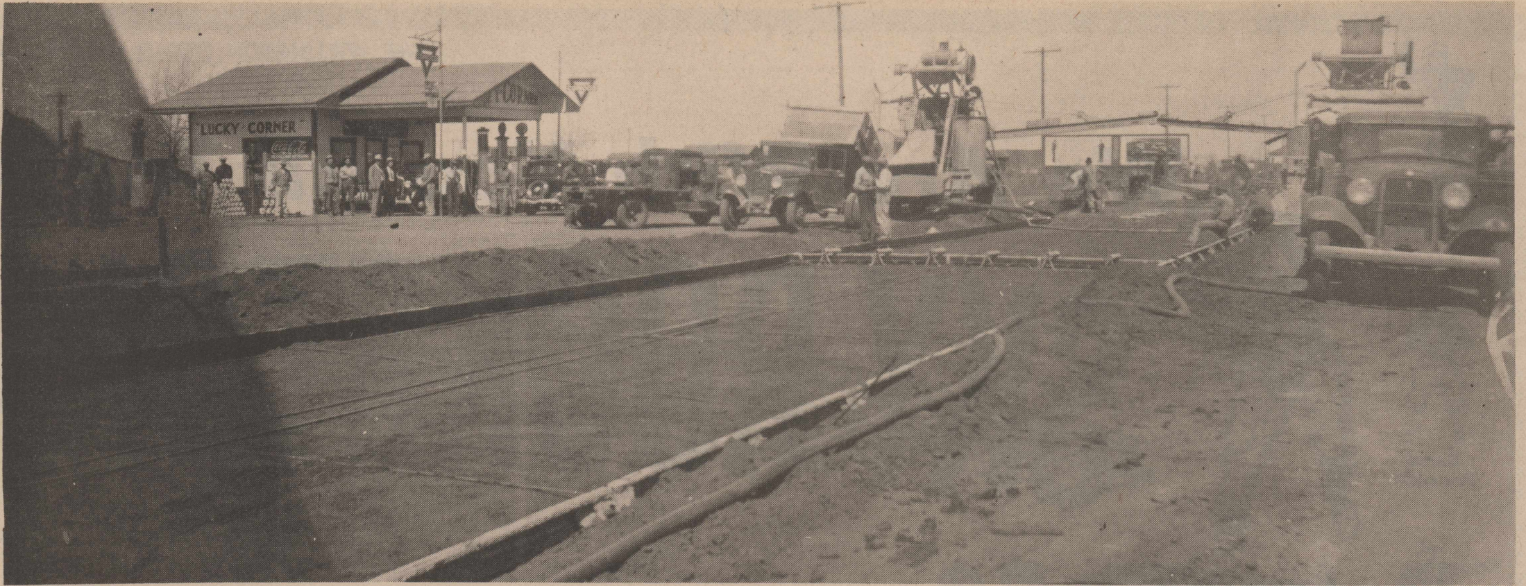
FIRST PAVED ROAD INTO WELLINGTON Concrete is poured into forms in early spring, 1936, at Lucky Corner, 15th Street and Hwy. 83, as the first paved
