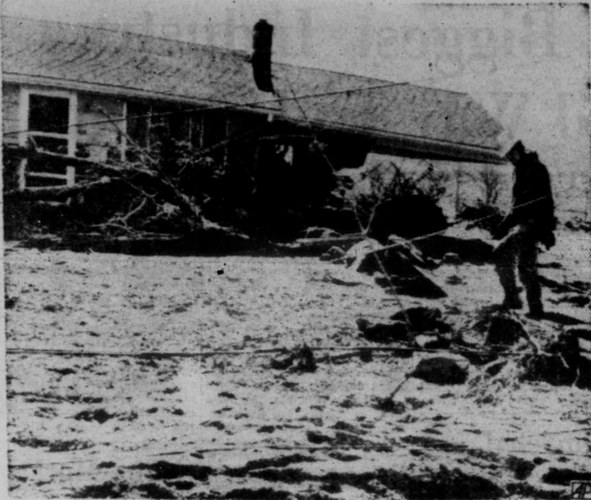
WATER POWER —The car port and part of the living room of a house show force of flash flood that tore through South Farms area of Middletown, Conn. A break in dam emptied Crystal Lake on residential area. (AP Wirephoto)
