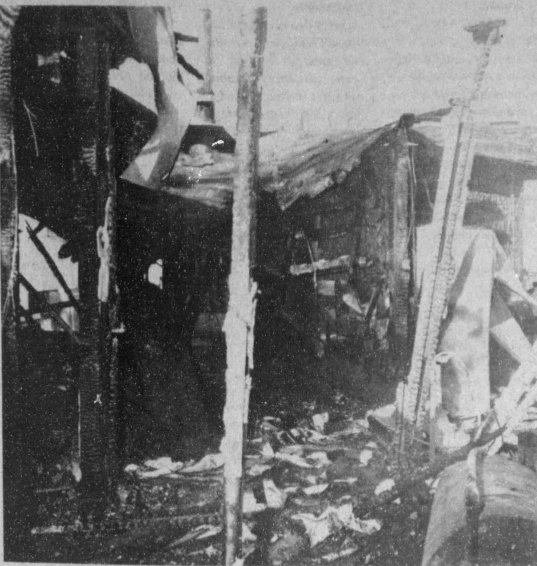
HOME GUTTED BY FIRE..... A fire of unknown origin struck at the Johnny Vaughn home in mid-afternoon on Sunday. According to reports, there was nothing salvaged from the blaze. Authorities have as yet been unable to determine the cause of the fire which also destroyed a small barn as well.
