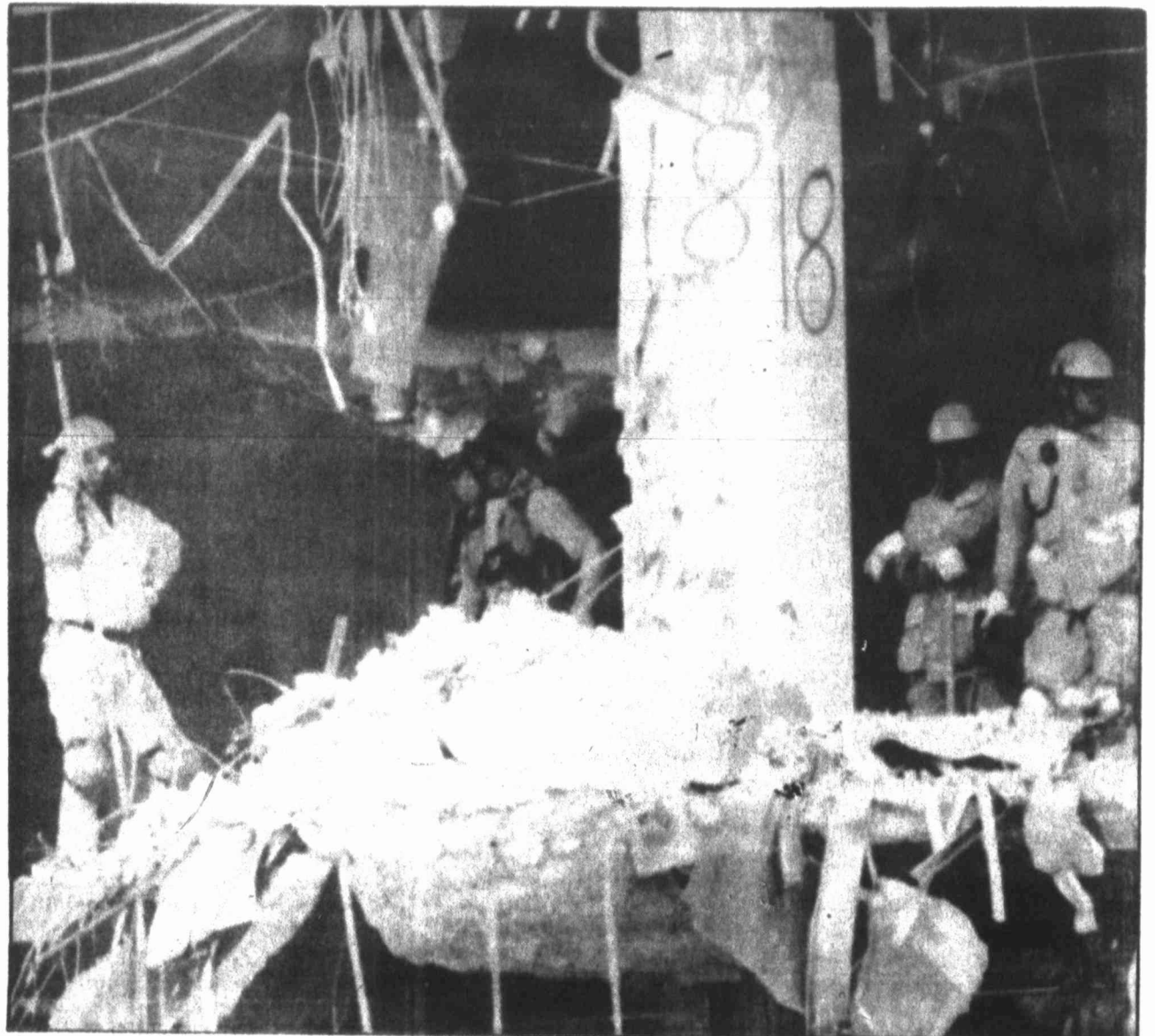
Rescue workers continue their efforts in the Alfred P. Murrah Federal Building in Oklahoma City on Monday as their shift ends. The nine-story building was bombed April 19. Late Monday evening, officials at the scene said they had removed three bodies, pushing the death toll to 83.
