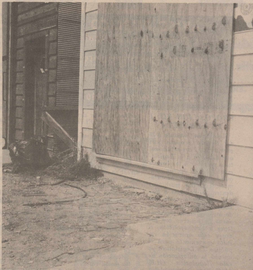
SITE OF NEAR TRAGEDY - Willie Diaz and Rodolfo Gonzales Jr. received serious burns Saturday when an explosion rocked Danny's Motor Service. In addition to this plate glass window being blown from the building, roof damages were also inflicted to the sheet iron shop.
