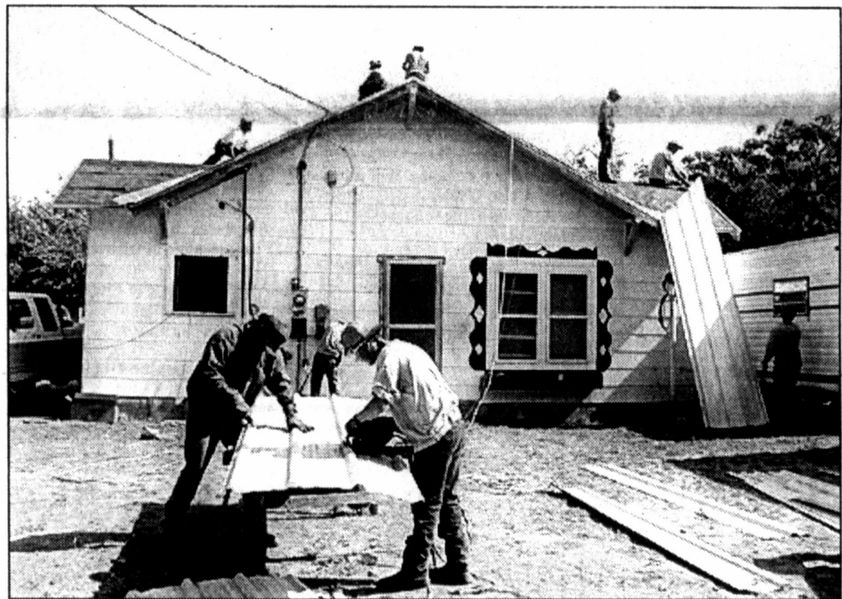
CHRISTMAS IN APRIL VOLUNTEERS, from left in front, Santos Ruiz Sr. and Calvin Hunter and, at right in back, Rusty Merket were hard at work Saturday at the Gene Martin house on East 11th Street. 150 volunteers finished extensive work on six Colorado City homes, bringing the program's eight year total to 174, and had only touch up work remaining on three of those houses this week. Photo by John Martinez
