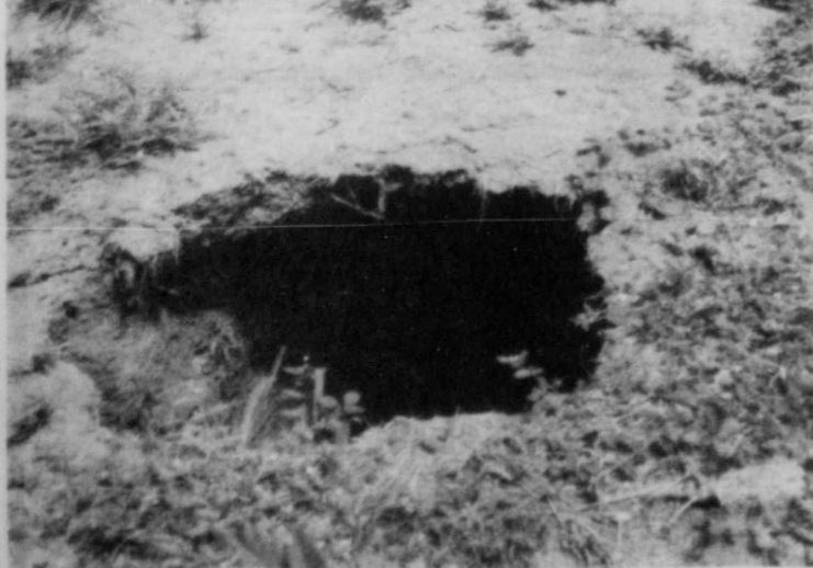
OPEN WELLS — Pictured above, are improperly covered abandoned wells. The well in the bottom picture has not been even improperly-capped. The cement block and casing have been removed, leaving a deep hole ready to cave in with any pressure — even the weight of the smallest child.
