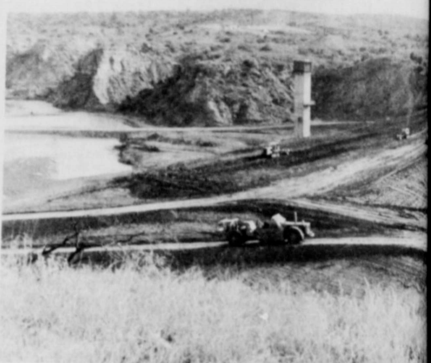
DAM WORK catches water that is used in construction of the dam at base and will be 28 feet on top. Highway on top of dam will
