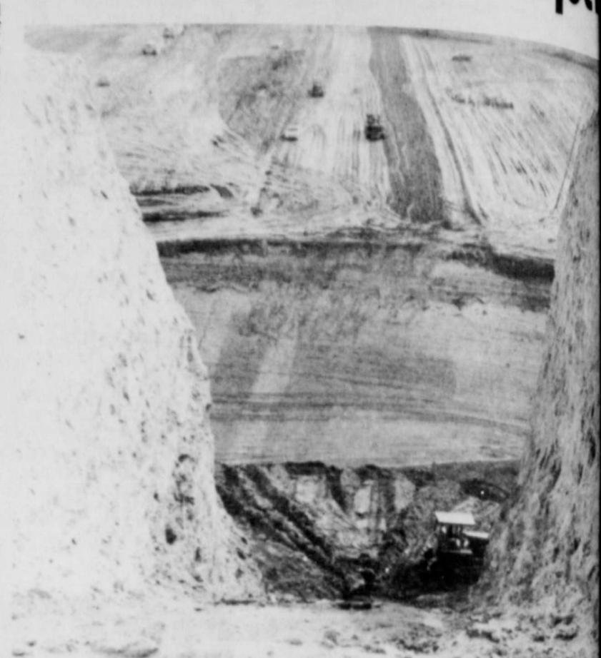
THIS SLASH IN THE EMBANKMENT will be filled with clay across the dam will go across it. . . dam building is in the background.
