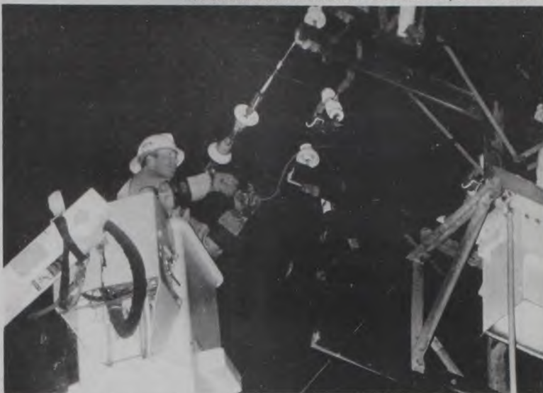
The Town of Lindsay experienced a two-hour blackout Saturday evening when high winds and tree branches snapped a power line downtown. At approximately 6:30 p.m., the downed line burned a jumper switch on Hwy. 82, causing the outage of the entire town. Services at St. Peter's Church were held using candles and lanterns. The restaurants served whom they could, with most businesses locking their doors until they were able to supply service when the lights finally came back on. TU Electric repairman Johnny Williams works to get the power back on. Janie Hartman Photos
