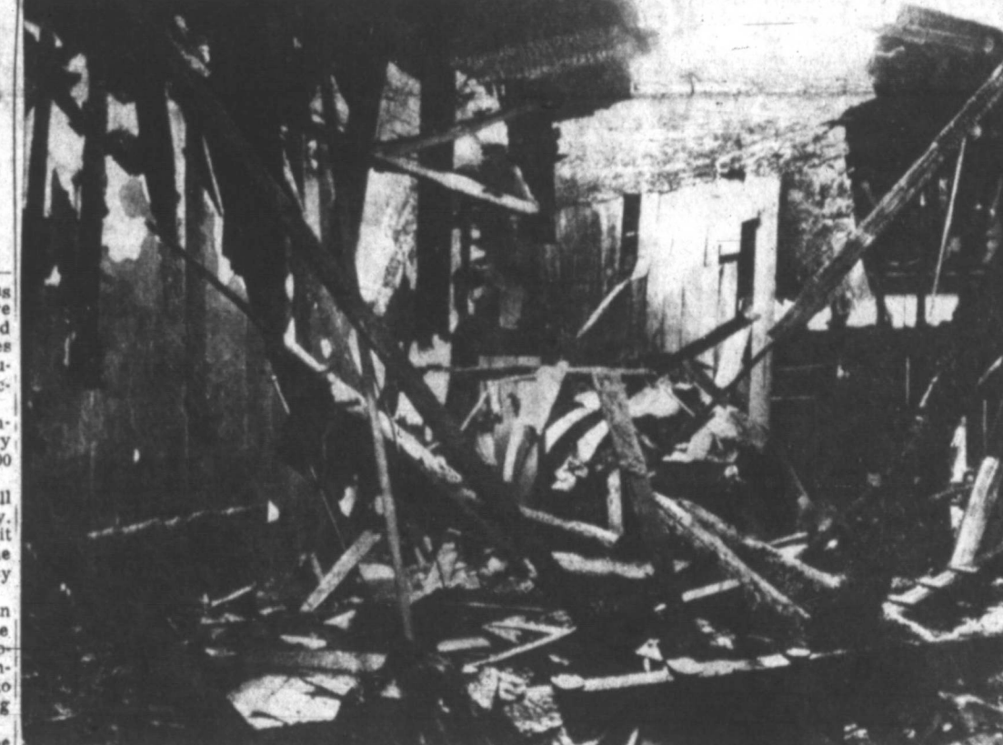
SHAMBLES — This was the rear of Enloe's Cleaners, 121 E. Kingsmill, this morning, following an early morning fire—worst in Pampa in six years—which raged through a five-concern area. In the rear of the picture are two doors, one on each side, about the only items in the store which were not destroyed. This was the aftermath of Pampa's $100,000 fire, burnt timbers glistening in the morning sun, trickles of firemen's water hitting what had been the floor.
