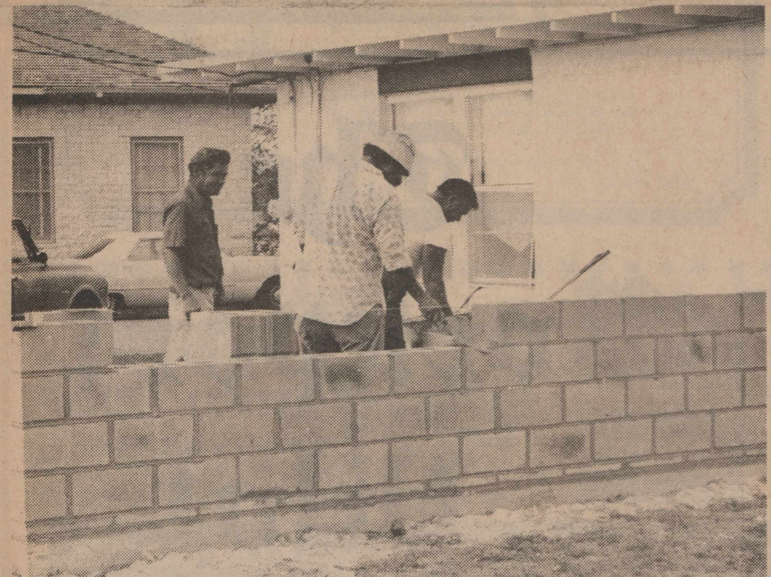
ONE BY ONE, THE BRICKS ARE PUT IN place for the new addition to the Rockport Chamber of Commerce building. The work began on the new wing last Friday morning.
