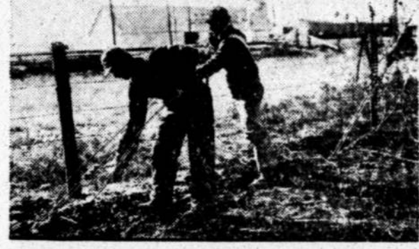
One reason why the giant poles of electric distribution and transmission lines can withstand the terrific strains that they do is because they are so carefully stored wherever possible. Here Mastel Wadkins and Wayne Gregston of Midland make secure the guy wires on a transmission line dead-end.
