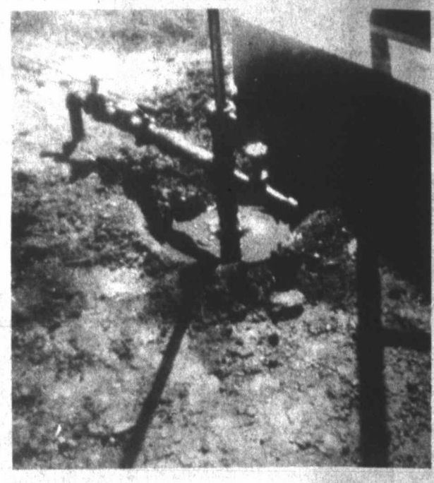
BUBBLING GAS and oil around this well indicates deteriorated casing at this well, at the Roy Bell farm.
