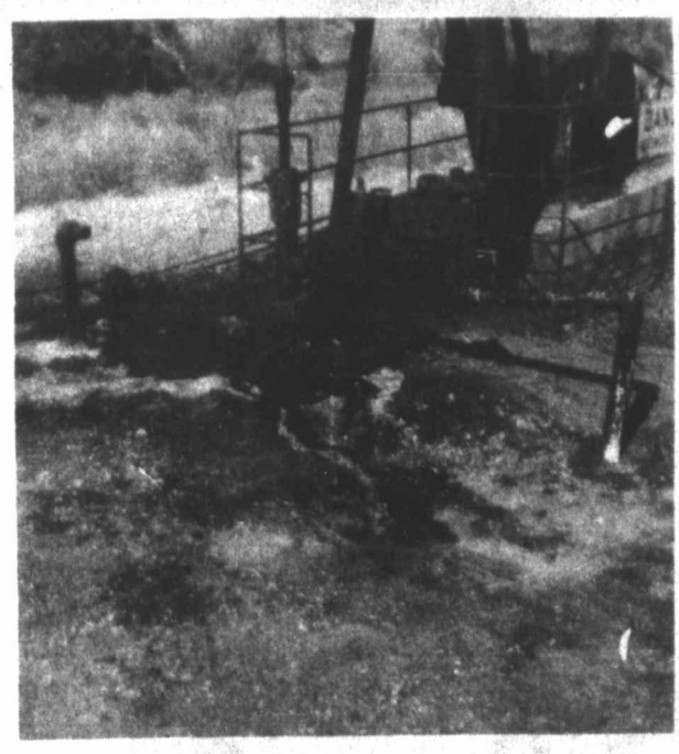
"OIL WELLS" pumping pure salt water, with chloride content of 150,000 ppm, leaking from the packing.
