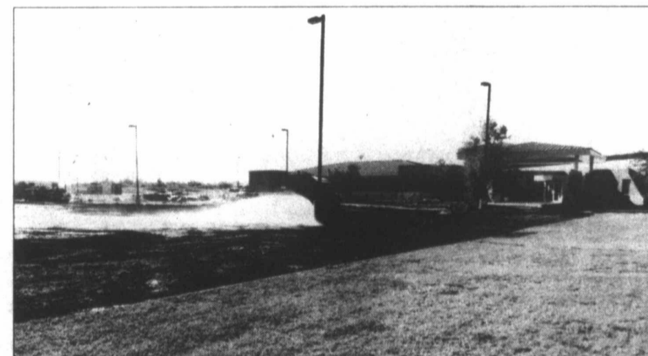
IN WITH THE NEW... The Mitchell County Hospital campus is getting freshly paved parking lots, and paving crews have been busy removing the old asphalt and leveling the dirt underneath in preparation for the new surface.
