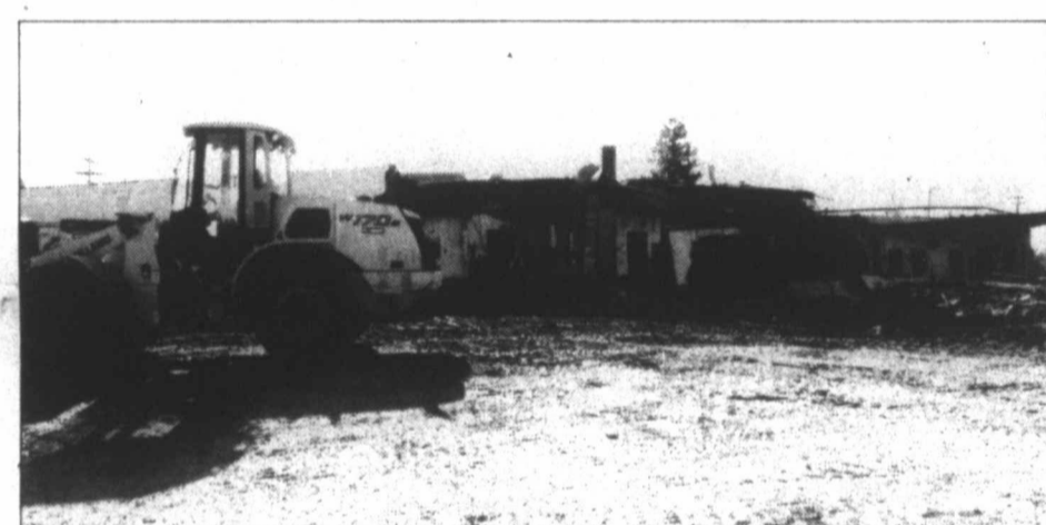
OUT WITH THE OLD... Crews from Ellis Construction are making progress on the demolition of the old Root Memorial Hospital building on Chestnut Street. Demolition began on the back side of the building, where the former emergency department was housed.
