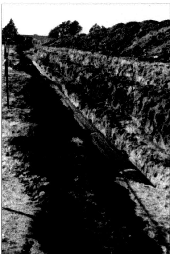
NEW DRAINAGE - 10th Street is closed and will remain closed for most of the week, so that 20" drainage pipes can be installed as part of construction of the new Colorado ISD campus.
