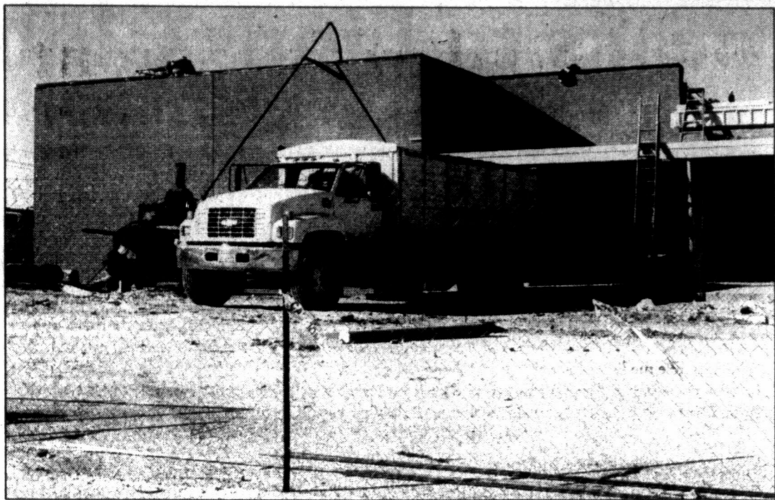
NEW DIGS - Construction and renovation on the Westbrook ISD campus is almost complete. Superintendent Todd Burleson said that he expects to be moved in to the new spaces in the next couple of weeks.
