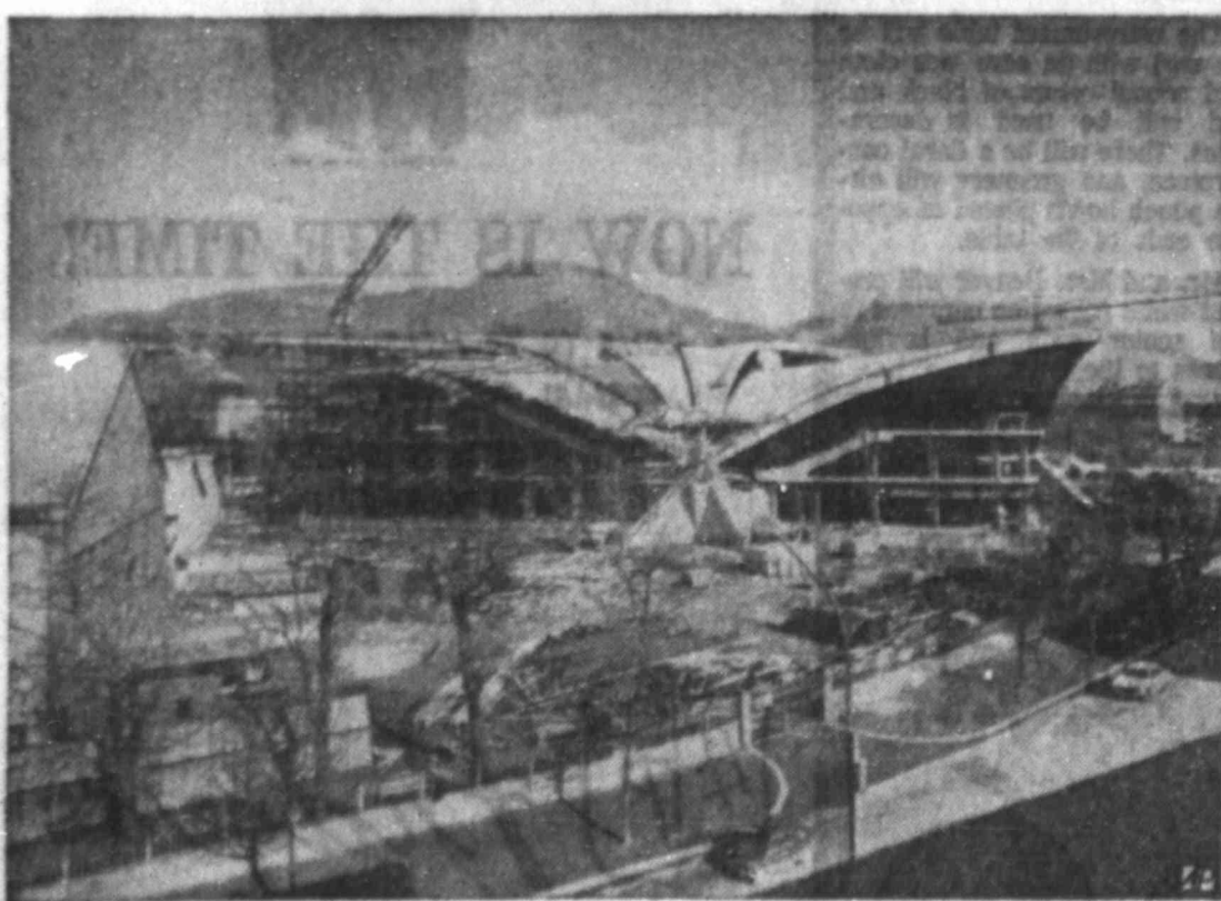
UP FOR NEXT YEAR — Work continues on the Ice Stadium that will house the skating and hockey events of the 1968 Winter Olympic Games to be held in Grenoble, France.
