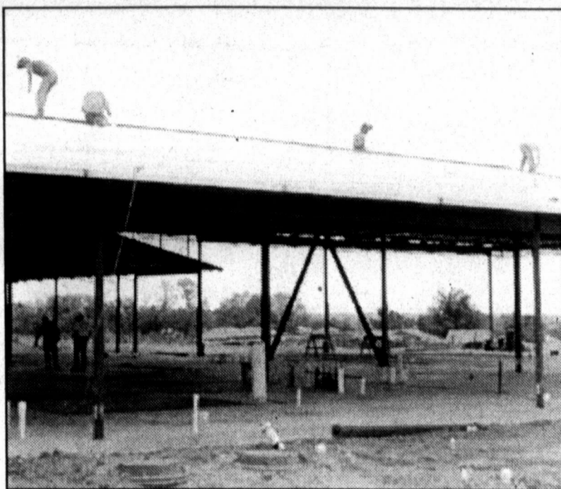
THE WEST SIDE ROOF OF THE NEW HOSPITAL was under construction Friday as workmen awaited the arrival of more roofing materials from Houston.
