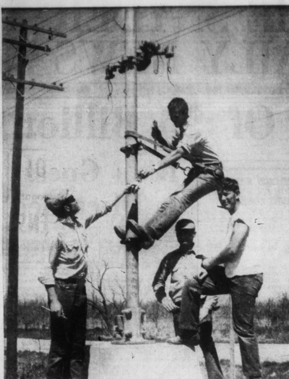
INSTALLING SAFETY DEVICE —This crew is installing warning signals at the Santa Fe Railway crossing of Huffman Street in North Snyder. The railroad is nearing completion of similar installations at all grade crossings here which were without warning signals previously.
