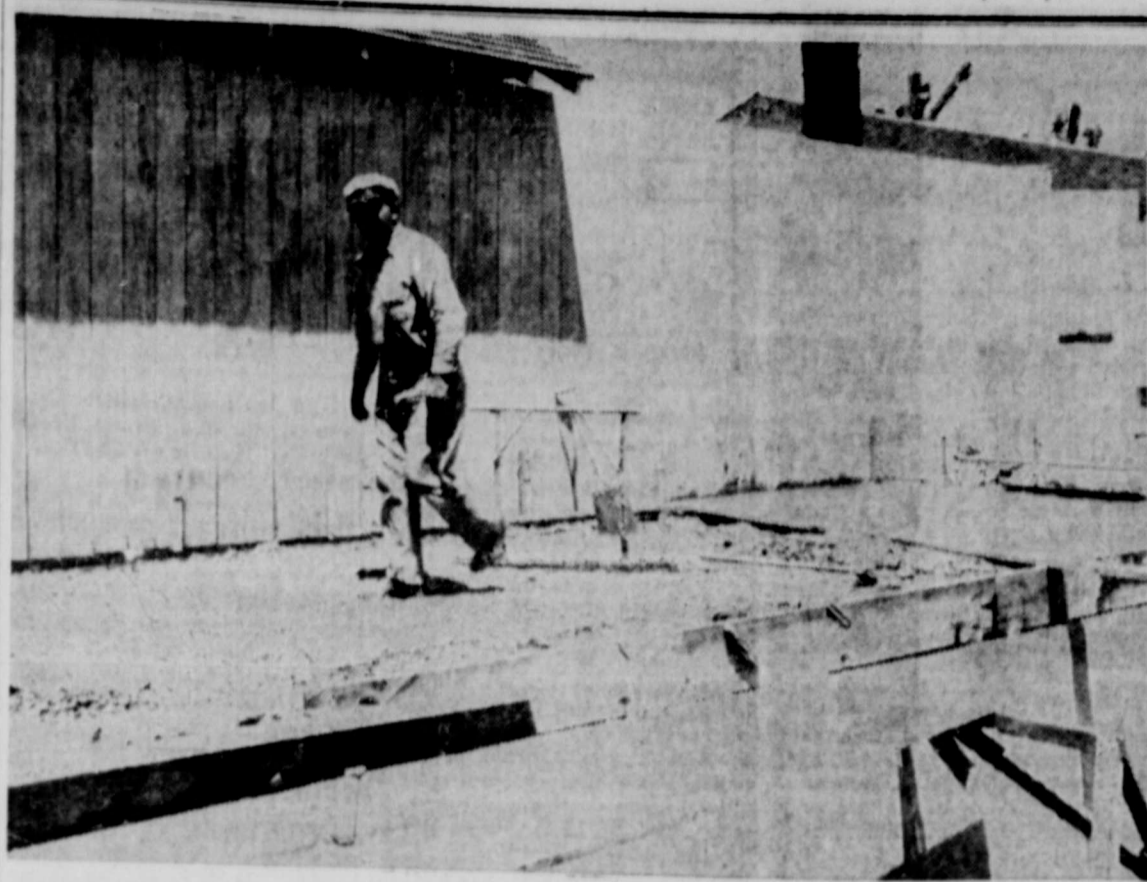
CONCRETE FOR SWIMMING POOL—Among the improvements being made at the Perryton swimming pool this week is the replacement of the runway at the south end of the pool with new concrete. Above is Johnny Ferguson, of the Ferguson Ready-Mix Co., supervising the pouring of the concrete. The pool will open next Tuesday.
