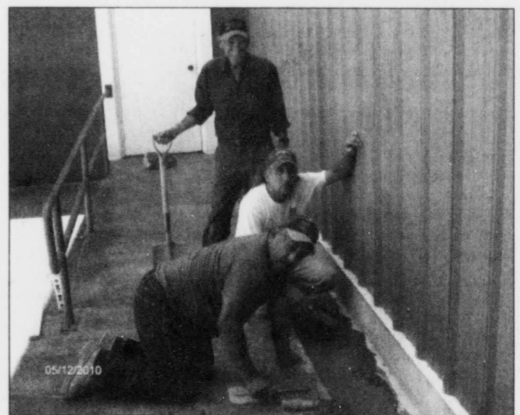
FINISHING TOUCHES ON the Opera House are cemented into place by (from back) Felix Franco of Franco Lone Wolf Concrete, Tony Gonzalez and Henry Rivera as they prepare the rain gutter for drainage in time for the concert by Jay Boy Adams on Saturday. Photo by Jan Lemons
