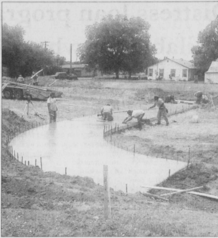
WORKERS ARE HALF WAY through with construction on the Vine Street extension. The new road will provide interstate access for the new Western Suites motel currently under construction. Photo courtesy City Hall
