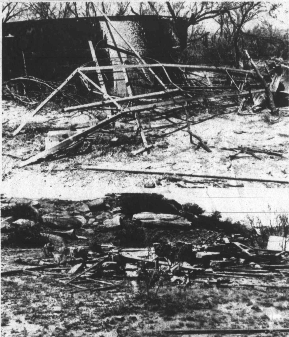
TORNADO DESTRUCTION on the Francis Winn ranch in southern Mitchell County Friday night completely wiped out a sheep shearing camp, including a windmill tower, shown in the top photo, and a two-room house and foundation, pictured at bottom. Also destroyed was a small shed and some sheep pens along with a lot of fence both in the immediate area and on other parts of the ranch.
