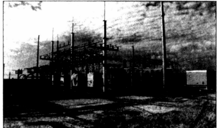
BETTER SERVICE? The new sub-station is being constructed two miles south of Loraine on FM 644. The facility is owned by Sharyland and will allow the company to tap into Oncor's major distribution line nearby. This will be a major upgrade for Mitchell County, according to officials constructing the project.
