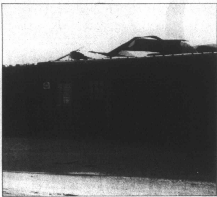
LOTS OF WIND, LITTLE RAIN – A storm cloud blew through Saturday evening bringing with it high winds but very little rain. Several areas of town were affected by the 60 to 70 mph winds, including Fort Wood, where metal roofing was curled up and part of the outer fence fell. Photo courtesy of David Arellano.
