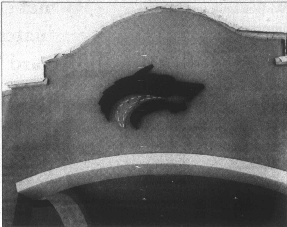
GO WOLVES! The exterior of the new multi-purpose building that houses a competition gym got a new look as a Wolf logo, which will light up, was beginning to be installed earlier in the week. Crews are working hard to get the gym ready for district volleyball games in October.
