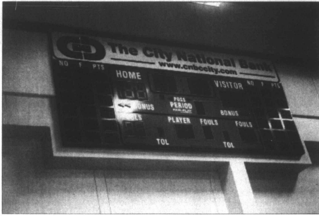
READY FOR ACTION! The new scoreboard was up and ready for some play in the new gymnasium that is being constructed as part of the new Colorado ISD campus. The multi-purpose building will also house a weight room, band hall and art room, along with the new competition-size gym.
