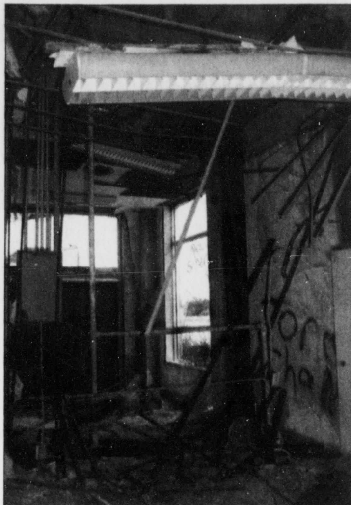
SAFETY ISSUES PROMPT city officials to removed broken glass, falling ballasts and floor debris from inside the Baker Hotel.
