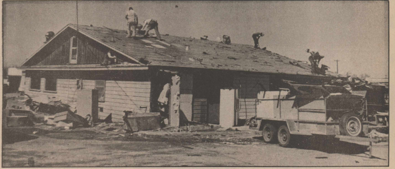
OPERATION "FACELIFT": Work crews have been busy lately remodeling this structure on Cleveland Street. The former restaurant will be home to Hargrove Crop Insurance. The facelift should be complete in thirty days.
