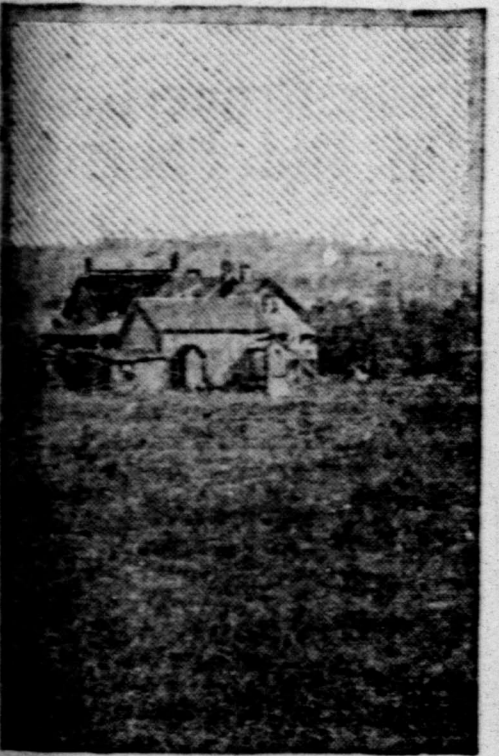
REAR PORTION OF THE HOUSE, CAUSING THE ROOF TO SAG. IN ADDITION THE OLD SHINGLES HAVE STARTED UP SO THAT THE ROOF LEAKS BADLY. IT IS ASSERTED THAT THE TOTAL REPAIRS NEEDED ON ALL THE BUILDINGS WOULD COST OVER $1,000.
