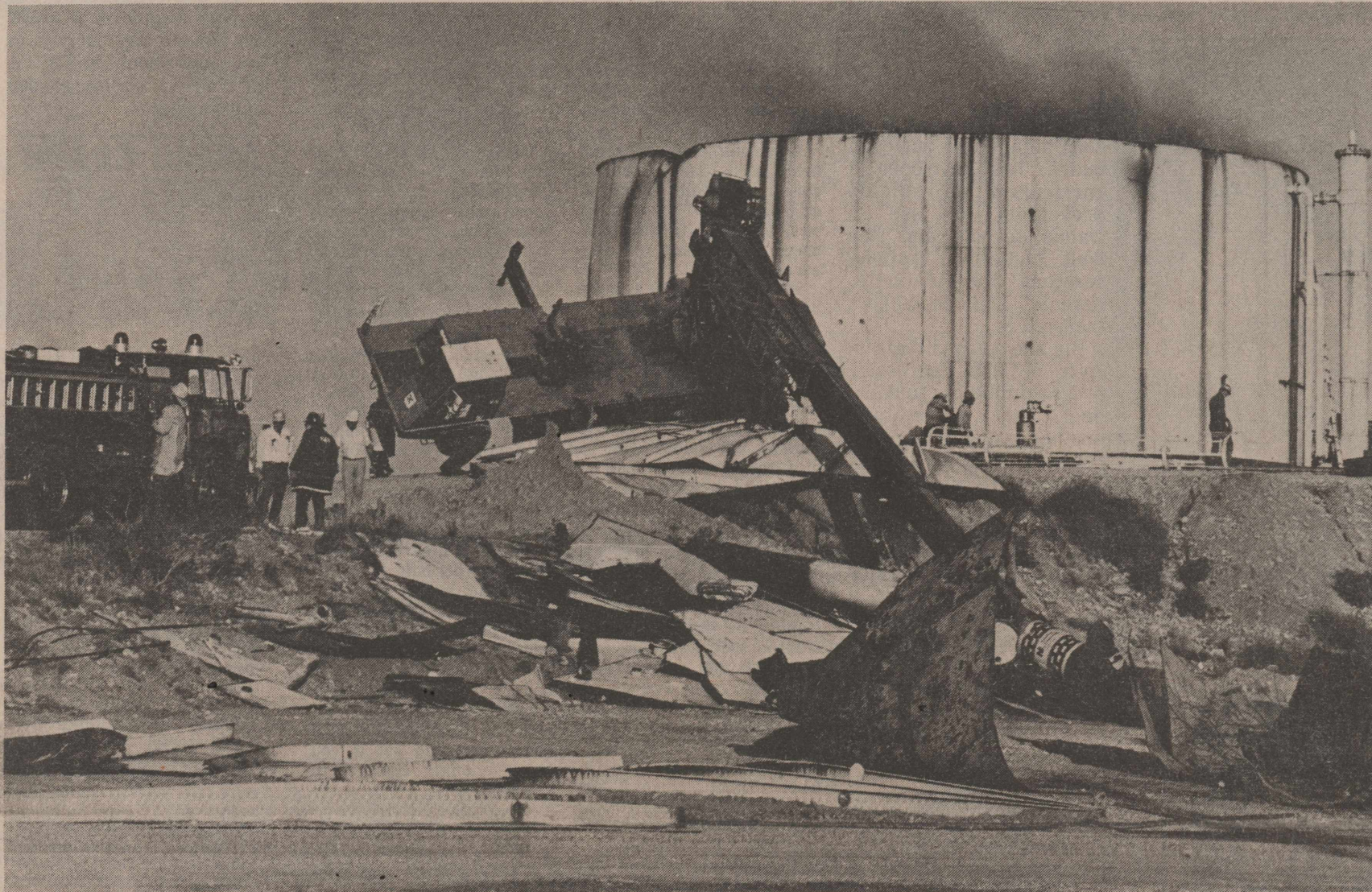
Toppled crane at fire scene Thursday afternoon (SDN Photo)
