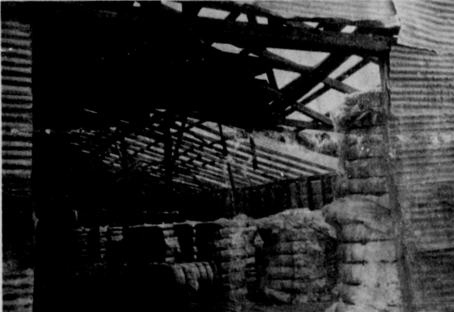
Inside View Of Destroyed Warehouse Roof
