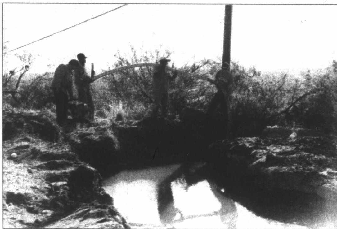
WATER, WATER EVERYWHERE - City employees (l-r) Nathan Slater, Jamal Green, James Walthall and Jordan Womack working on a water leak on South Hwy. 163. City crews worked through the night Monday to contain the leak in the 16" pipe.
