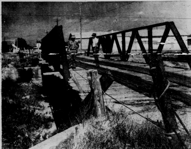
DANGER, BRIDGE OUT! —Supports have rotted and fallen away, railings have disappeared with the years, and there is no longer any solid structure on which to put repairs on the old county bridge over Deep Creek on Twenty-first Street. With no possible way of making repairs and making the bridge safe, the city council decided that with the help of Precinct 2 Commissioner Bill Herring, the city would construct a new bridge. Above, City Engineer Bill Kimzie and City Manager Roy Dunlap look over the structure in preparation to starting tearing it down. The bridge has been closed for weeks.
