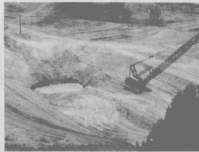
This trench that was dug recently at the Palo Duro Dam site immediately filled itself with water.
