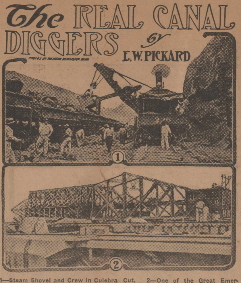
1—Steam Shovel and Crew in Culebra Cut. 2—One of the Great Emergency Dams Devised to Protect the Locks.
