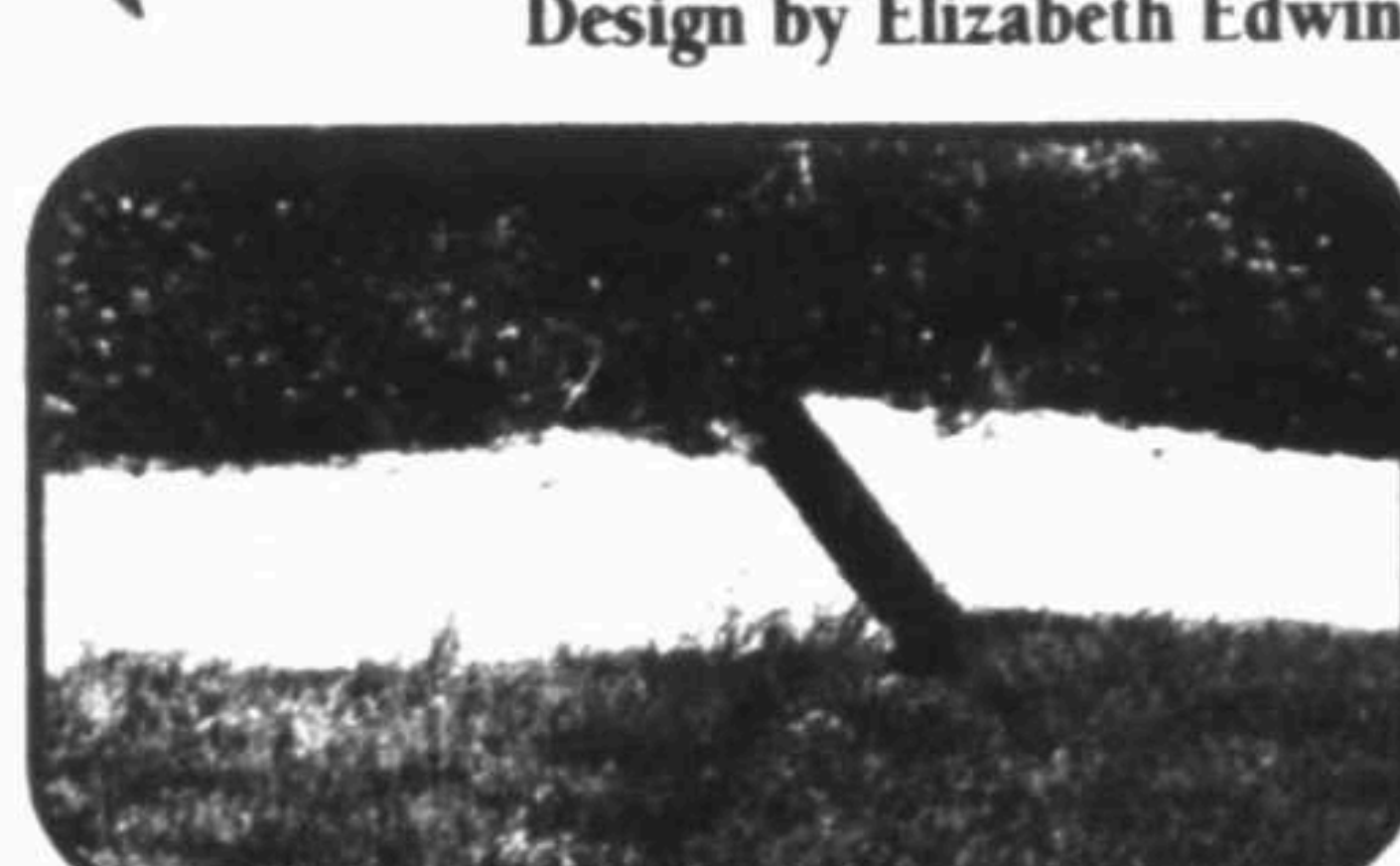
Tree species with shallow invasive roots can heave and buckle sidewalks, patios, drives and curbing, creating a safety hazard.
