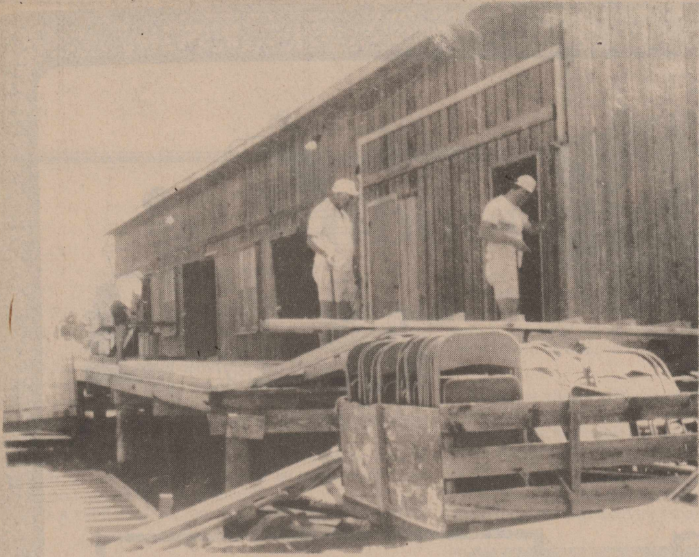
HANK KOPFLOW, MICK LADNER and Jerry Ladner are among the volunteers who helped remove furniture and appliances and dismantle the back porch of the Paws & Taws Building this past weekend in preparation for moving the building to Fulton Park. In the foreground, a trailer full of chairs awaits transportation to storage. The move has been delayed and is now scheduled for some time during the week of July 4.
