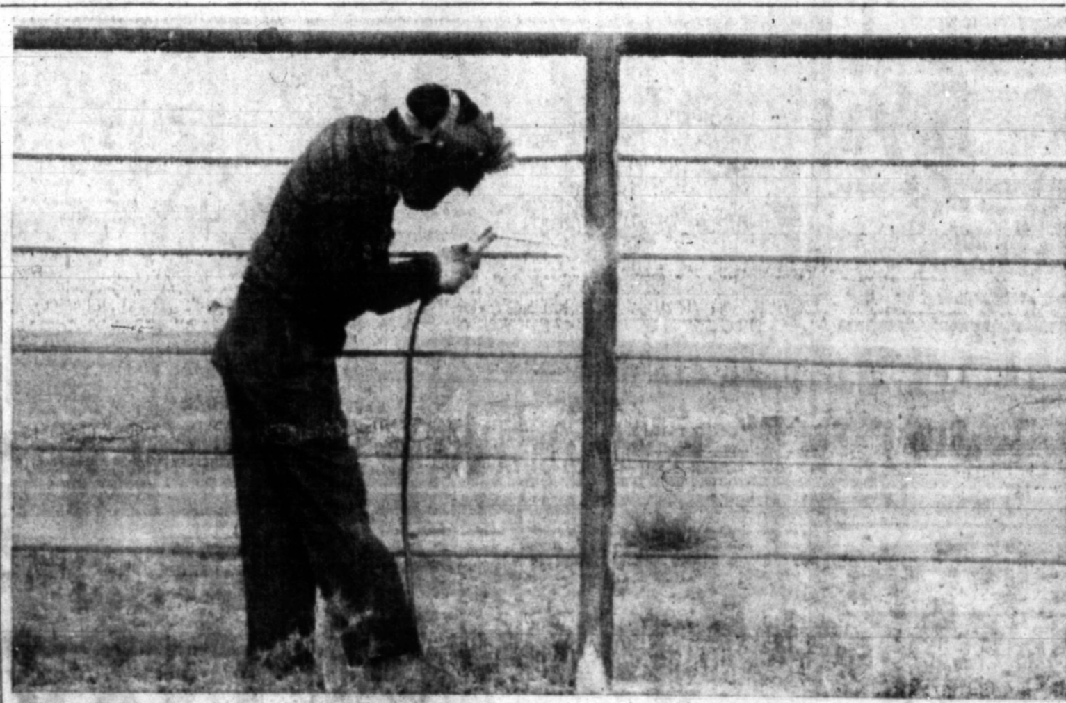
STEEL MAKES A DANDY FENCE — Odell Fryer welds steel rods into upright posts to strengthen a new steel fence being built around the V. E. Wagner residence at 504 N. Price. The fence includes posts set in concrete with a two inch steel pipe across the top.
