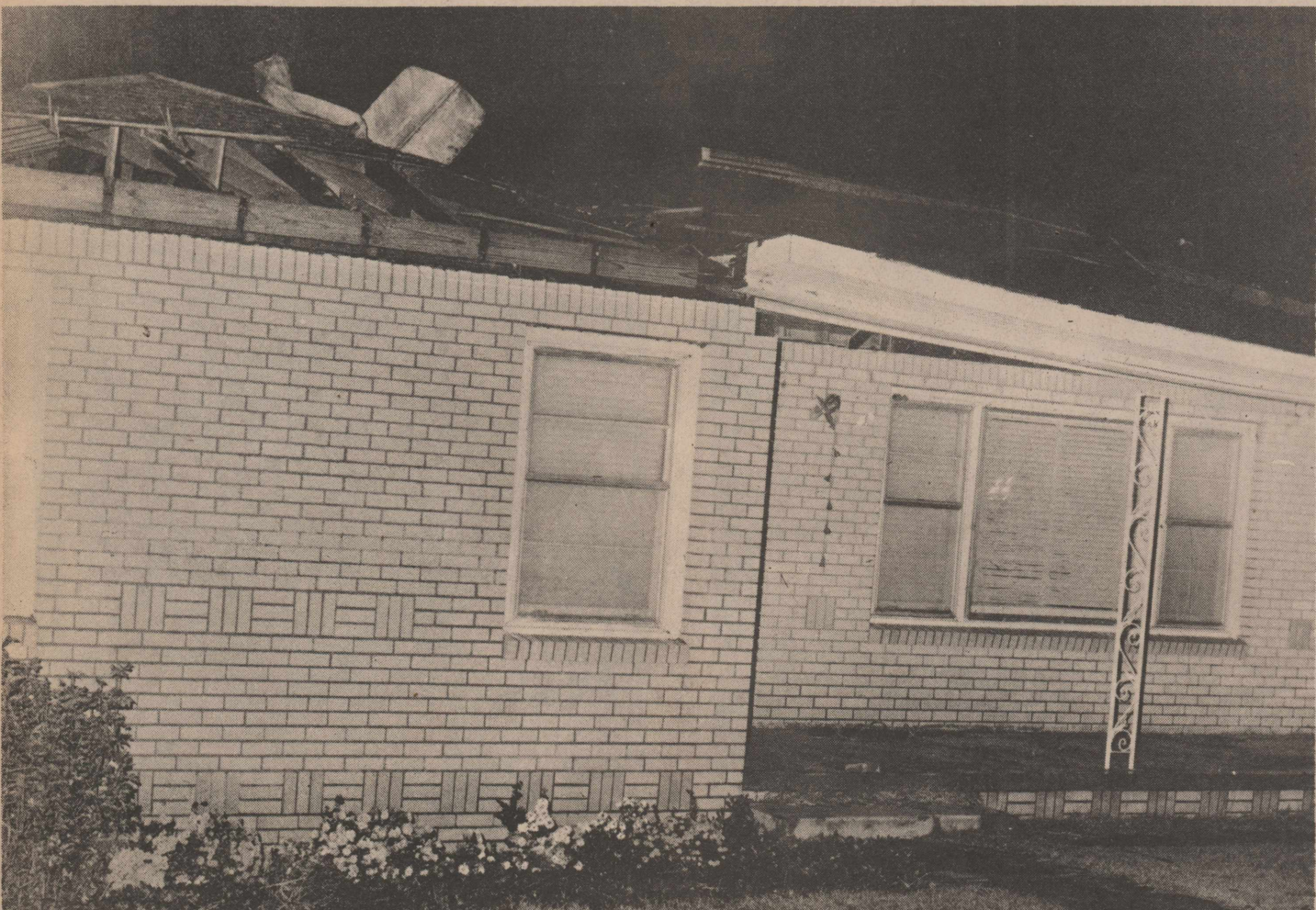
EAVES RIPPED UP AND ROOF TORN AWAY -- this is the west end of the Raymon Carson home after being hit by a
