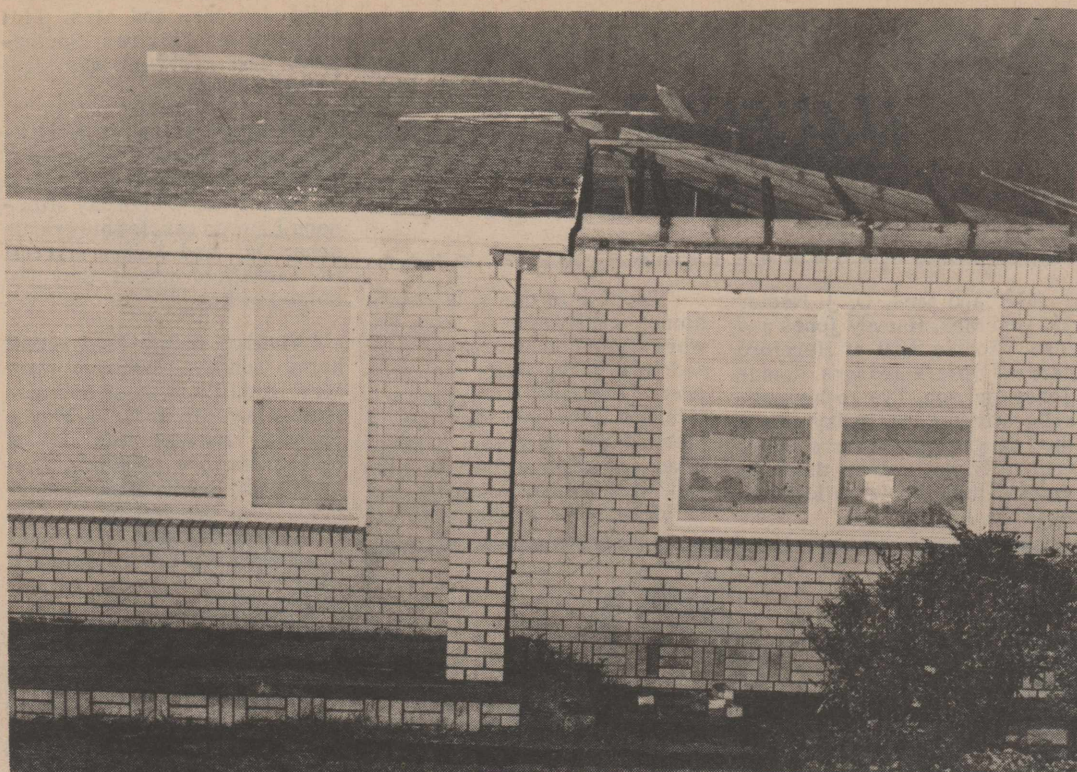
TORNADO STRUCK RAYMON CARSON'S HOME and took with it portions of the roof. Shown here is the east end of the house, where the roof was lifted and carried out into the field. Billy Carson was standing in the room shown here when the wind blew out the windows. He suffered minor cuts on one arm. (STAFF PHOTO)
