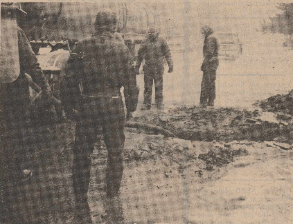
BOTH CITY officials and city employees spent many hours in sub-freezing temperatures last week finding and repairing broken water lines. The ground was frozen to a depth of 10 to 14 inches. Knox City was one of many area towns kept busy in checking water lines and meters.
