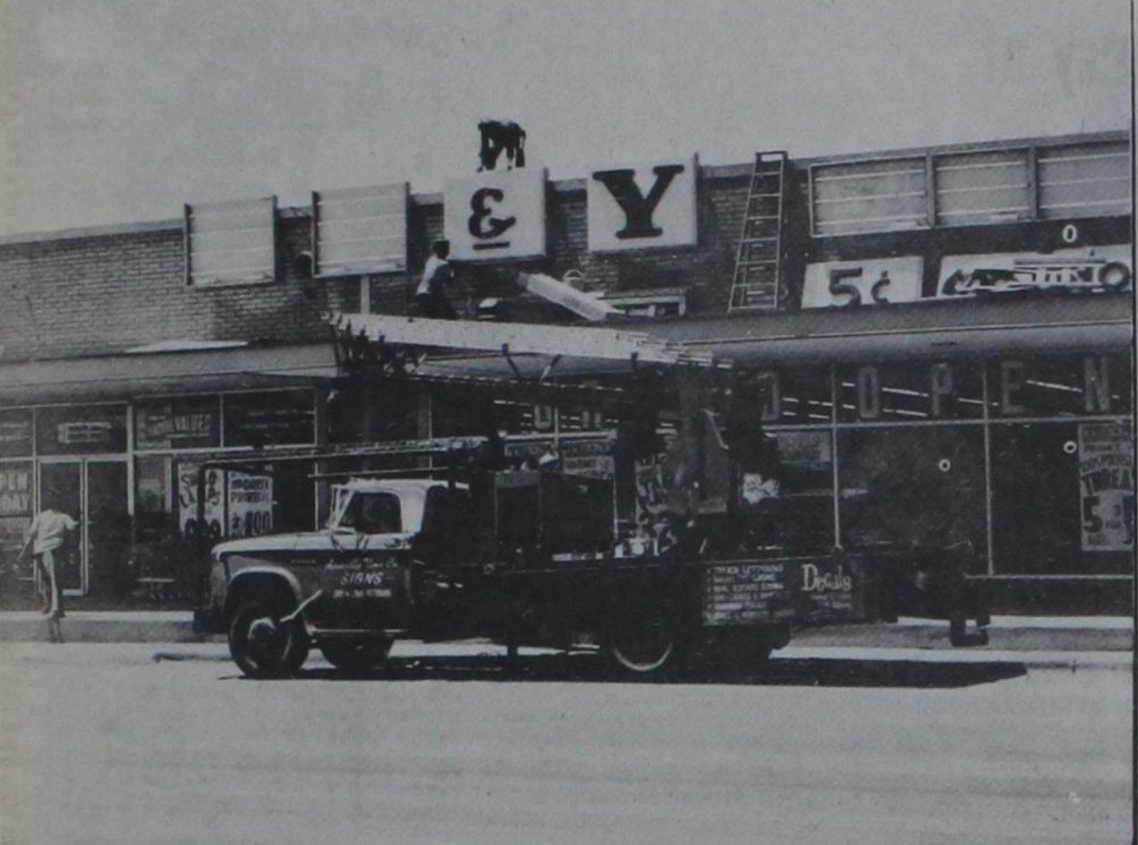
NEW SIGNS GO UP—Workmen were busy installing new signs at the front of the expanded TG&Y store here last Thursday. Work on the new lights is expected to be completed sometime this week when wiring is installed.
