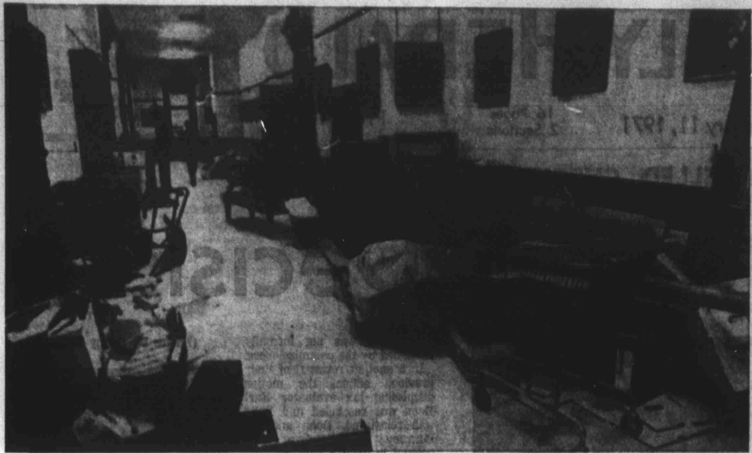
LITTERED HALLWAY AS SESSION NEARS — This hallway behind the senate chamber and leading to such offices as that of the lieutenant governor and secretary of the senate is littered with furniture, papers and an assortment of trash as workmen rushed to complete the task of getting ready for the opening of the legislature Tuesday.
