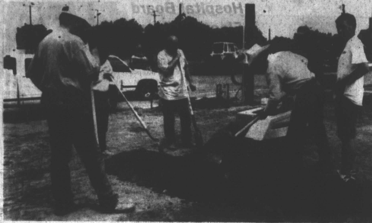
LOTS OF HELP - Many volunteers worked long hours Saturday to help put in a new sprinkler system at the Life Enrichment Center. Shown here (clockwise from left) is Greg Henley, Wes Owens, Joe Hays, Barry Pittman, David Ehlers, and Clay Pittman. (LCN PHOTO)
