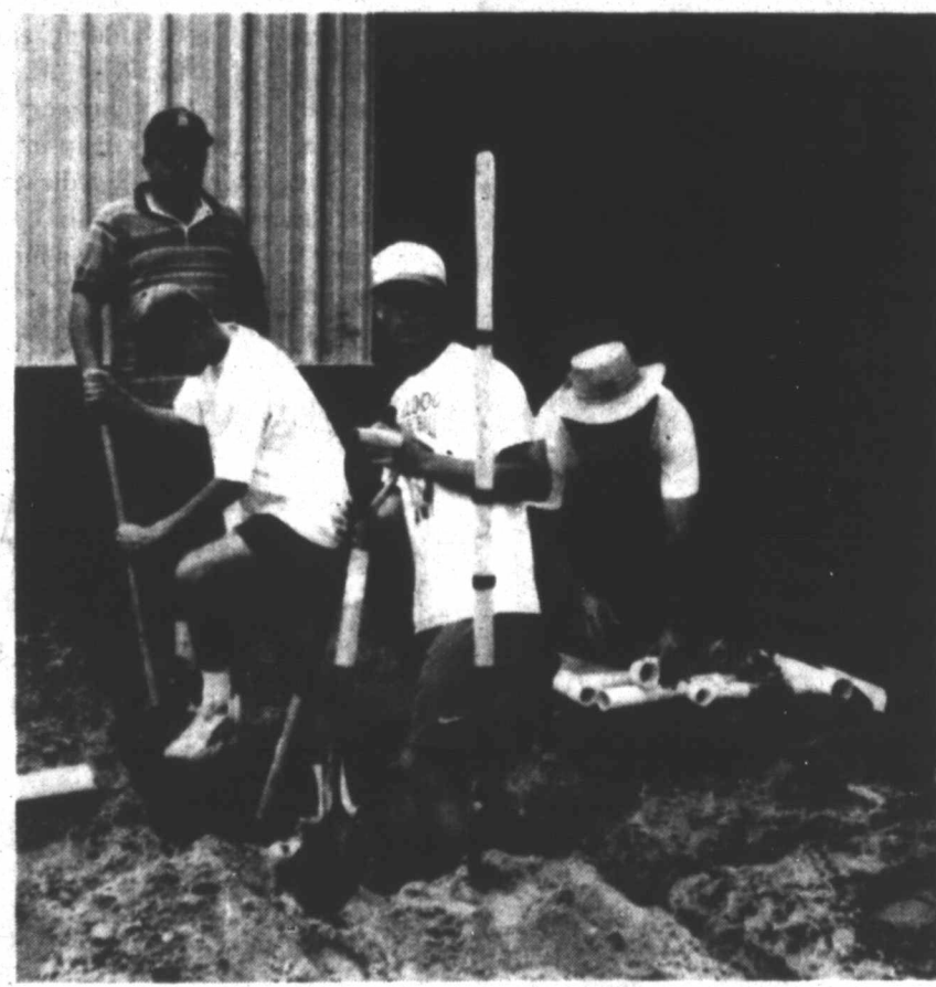
DIGGING TRENCHES - Volunteers leaded helping hands, as well as their feet and strong backs to help install the new sprinkler system at the Life Enrichment Center in Tahoka Saturday. Shown here are Tahoka Police Chief Steve Chance (standing), Brady Raindl and D.J. Sims in the ditch, and sorting pipes is THS Principal Jimmy Parker. (LCN PHOTO)
