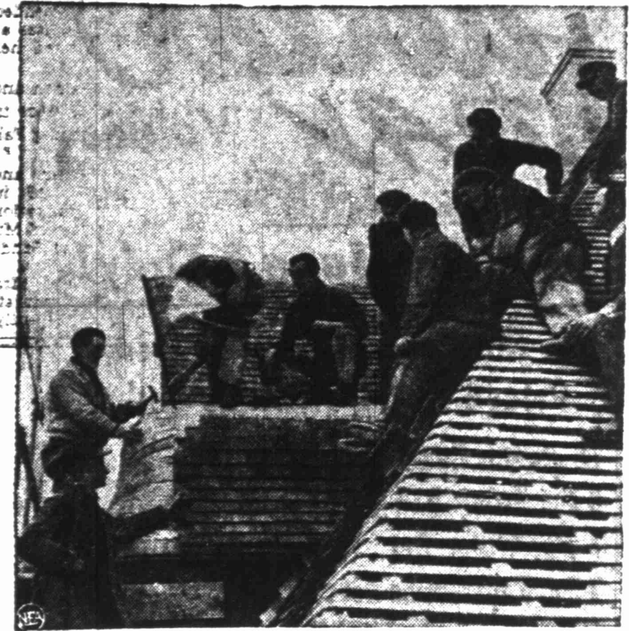
Under the rooftops of Paris could be plenty of living space to help in the current housing crisis. But under the rooftops also are lots of leaks; most of them need an army of workmen like this to make the once-romantic "garrets" livable.
