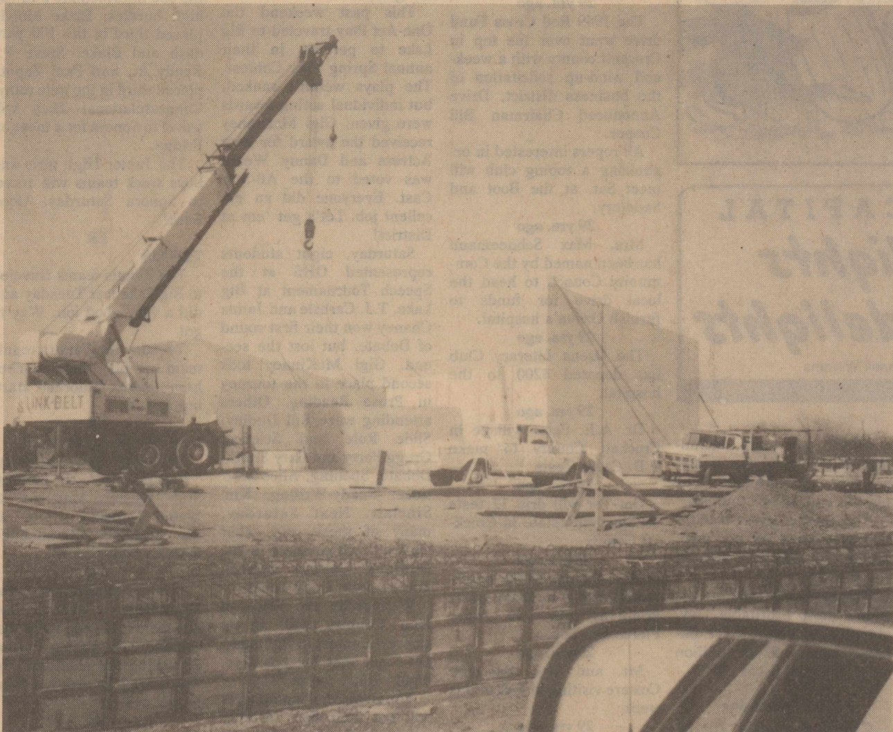
CONSTRUCTION IS MOVING RIGHT ALONG as scheduled in the school building program. Here the walls go up for the new elementary school which is being built across from the teacherages adjacent to I-10. Although looking like pre-fab material from a distance, they are far from it. The walls are pre-cast concrete shot through with steel and finished on the outside with rock.
