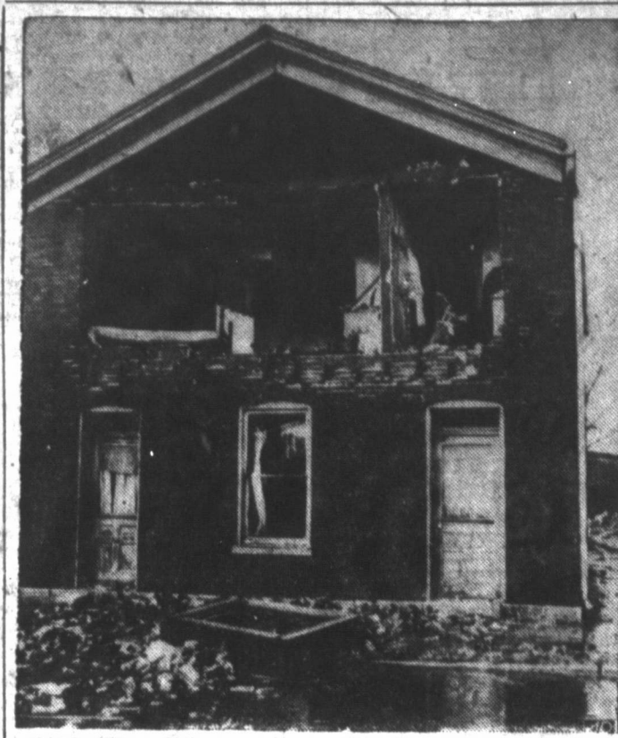
WINDSTORM DAMAGE—Second floor rooms of this Hannibal, Mo., building are exposed to the elements after a windstorm of "torrid proportions" swept through the northeastern section of the city. A number of buildings were badly damaged and three persons were reported injured. There were no deaths reported. (AP Wirephoto)
