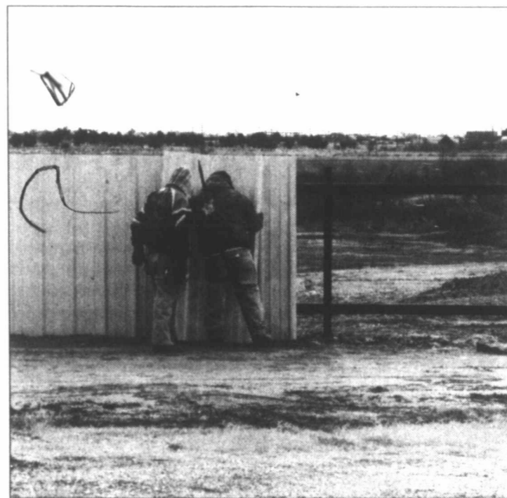
FENCING FOR SAFETY —A sheet metal fence was being installed last week by workers with Champion Creek Farms, LLC along 10 th Street near the new school. The fence will provide a barrier between 10 th Street and the pit from where dirt was taken to build the new CISD campus. It may also reduce the temptation for kids to go onto the property.
