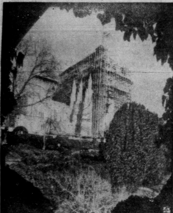
TOWER FRAME — The south transept of Washington Cathedral in the nation's capital is enclosed by steel scaffolding as work continues on a 300-foot high tower.
