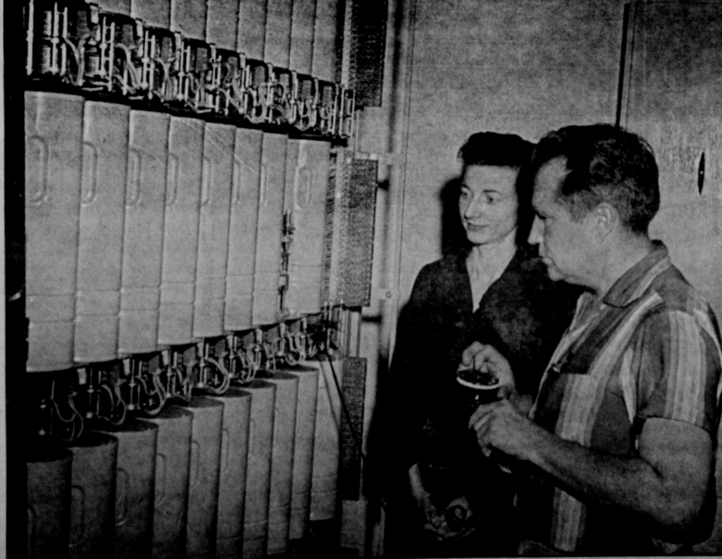
TELEPHONES ON INCREASE—Figures from Southwestern Bell Telephone Company here indicate that Slaton is growing steadily. In April 1951, total number of telephone instruments in use here was 1,394. In January of this year, the number had increased to 1,883. Pictured above are Miss Dorothy Jones, service representative, and H. H. "Soapy" Gore, plant manager, as Gore was running a check on some of the dial equipment here. (SLATONITE STAFF PHOTO)
