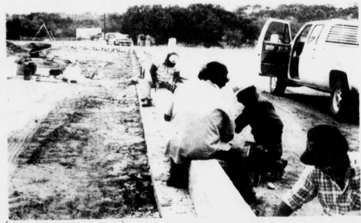
EXTENSIVE WORK is going on at Hutchinson Elementary School. Here workmen are putting up a retaining wall around the building.
